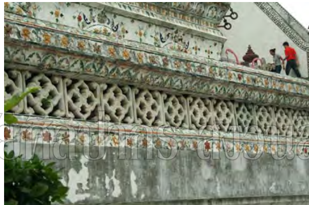
Figure 110: The wall of Phra Prang base showed sign of seepage by dampness causing decays
