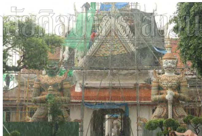
Figure 86: The restoration of the Entrance Way with Spire Roof in King Rama IX reign
