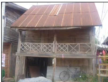
Figure 48 Two-story wooden house, attractive structure if repaired Source: Photograph taken by author on February 26, 2011
