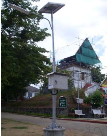
Figure 106 A solar cell electricity post (under the project of environmental conservation) used in Wat Phra Maha That: It is the one public place that uses environmental friendly lamps. It should be encouraged for practice at many more public, private, and household applications to lessen the environmental burdens.
