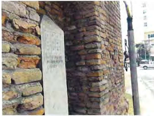
Figure 84 : Suan Prung Gate, Chiangmai City Wall, by the author on 19th March 2011
