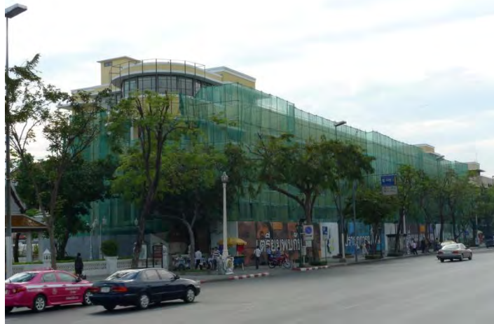
Figure 274: The site of “Nitas Rattanakosin” when it was under construction. This photograph was taken on 25 February 2010. Source: Naratuschan N.
