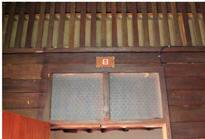
Figure 223: The signage of the room number over the old style windows, Source: Narin N.
