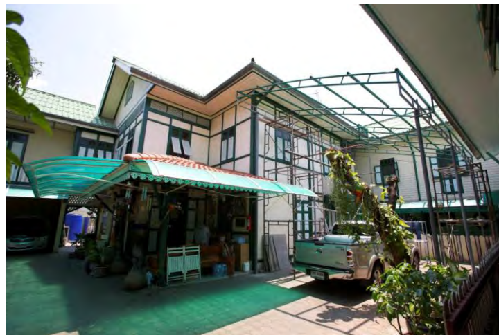
Figure 48: The extended structure has been built into the space between two buildings, a house of the owner and a remaining renovated guesthouse, Source: Naratuschan N.
