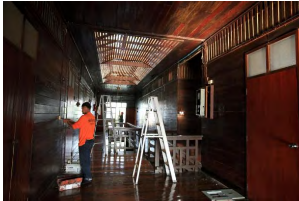
Figure 228: The 3rd floor of the Nanfa was the first to be renovated, Source: Narin N.
