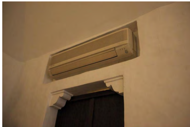
Figure 265: The intention to void some parts of the wall to place the air-conditioner helps to blend it, Source: Narin N.
