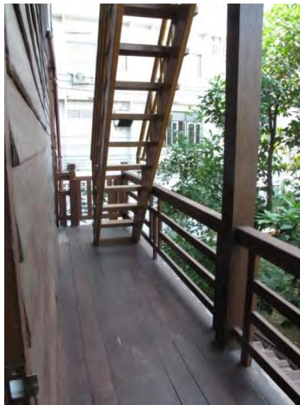
Figure 206: Compared with the figure 205 above, the Fire exit made of timber is located at the same place and seems to be a structure that remains unchanged, Source: Suparee B.
