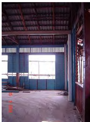
Figure 230: The floor was not covered or protected by any materials, Source: ibid
