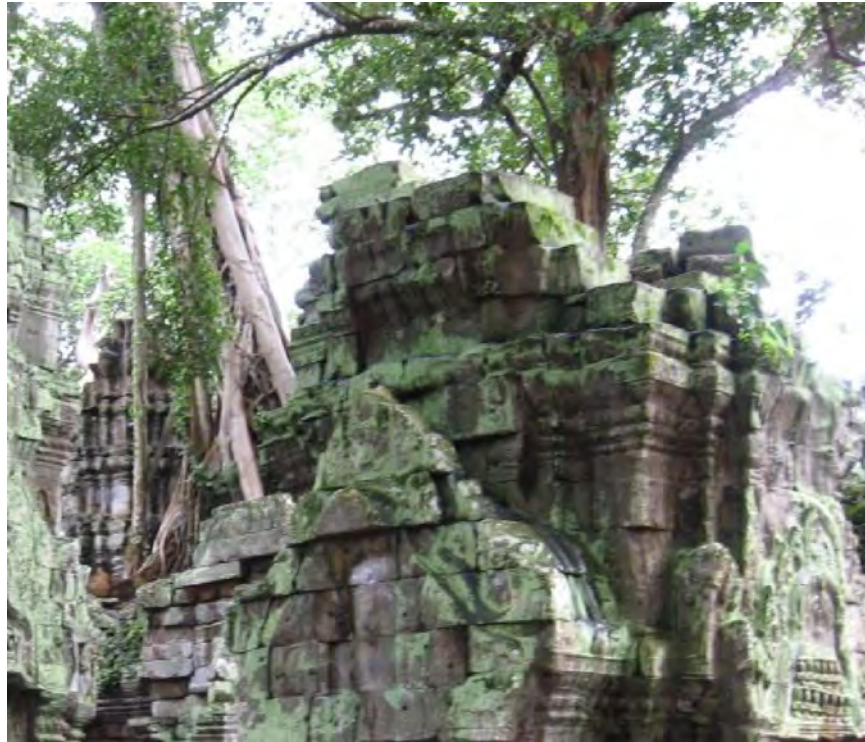
Fig. 41 The deterioration of the cultural heritage Prang as Buddhist Sanctuary Ta Prohm temple from root fig tree and lichen at the surface of the stone.
