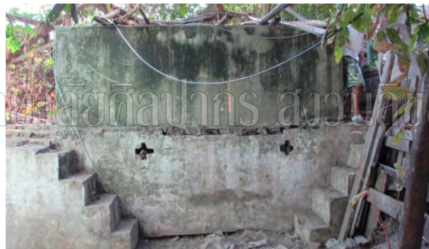
Figure 128 There were three layers of settlement wall used for protection. This is a second wall remaining after the outer wall collapsed into the river. Moreover, people brought bricks for their own proposes. Photograph by Phungwong, N. on October 21, 2011.
