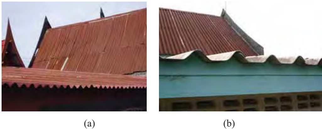
Figure 80 Roofing in the intermediate group: (a) Corrugated metal sheets and (b) Corrugated concrete tiles
