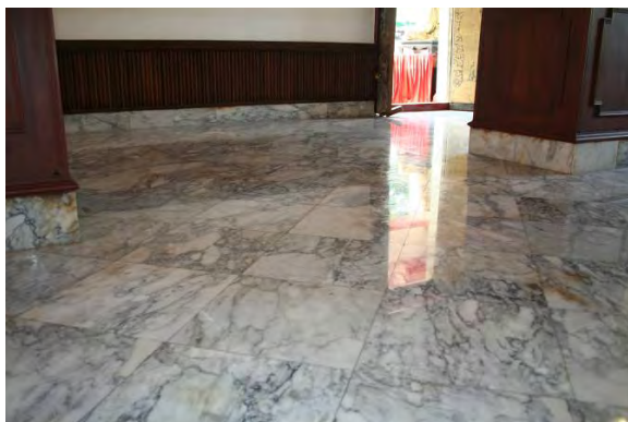
Figure 98: Marbles are used to be new materials instead of the old tiles for Viharn-noi or the small chapel restoration
