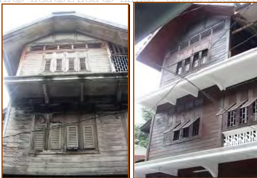
Figure 25-26: Front view (left) pictured in 2003 before repair, (right) pictured in 2010 Source: (left) provided by the Old Market Committee, (right) site survey, Aug 2010.
