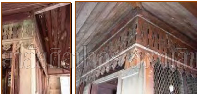
Figure 29-30: Ginger bread curtain 3 rd floor (left) pictured in 2003 before repair, (right) pictured in 2010
