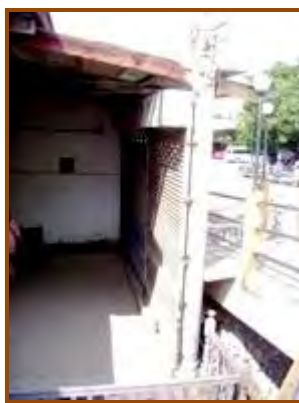
Figure 242: A gate to a main street is permanently closed
