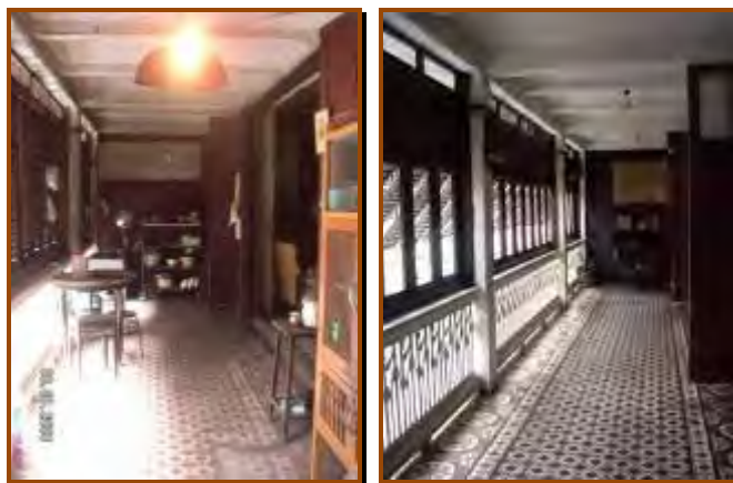
Figure 27-28: Corridor at 2 nd floor (left) pictured in 2003 before repair, (right) pictured in 2010
