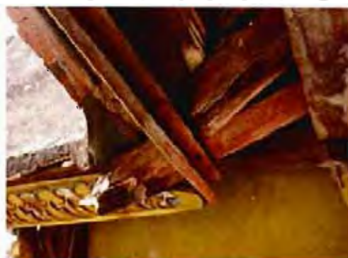
Figure 9: Under roof valley in decayed
