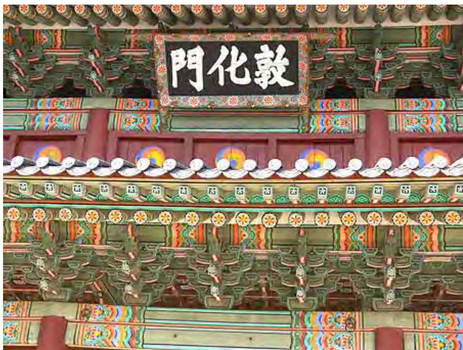
Figure 140: Name plate and roof decoration of main gate, Changdeok-gung (Photo by: Noh, Jang Suh)
