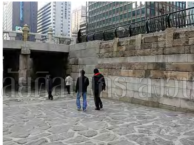
Figure 29: Retention wall near Gwangtong-gyo (Photo by Noh, Jang Suh. showing mixture of ancient stones and modern material)
