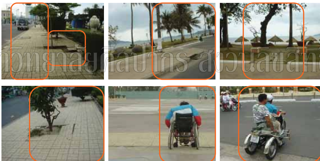
Figure 298: Nha Trang city sidewalks liking the trees outside, Sidewalks have been damaged by tree roots. Bushes and low tree branches upon the walkways make walking difficult along sidewalks. Obstacles on existing sidewalks can make walking difficult and sometimes dangerous to pedestrians who use wheelchairs.
