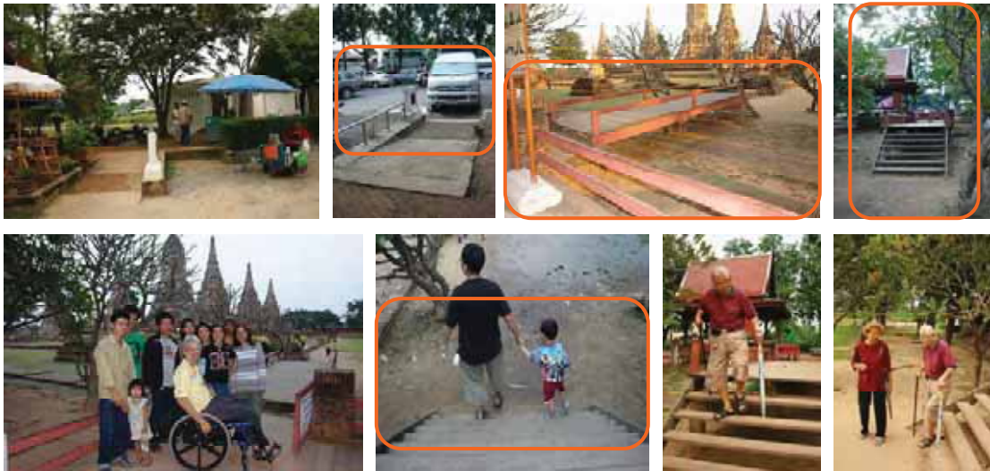
Figure 214: Ramp at the entrance and combination of toilet cubicles into one. Ramp does not have handrails. It should be provided for persons with mobility impairments and elderly.
