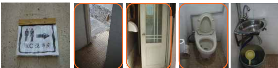
Figure 173: Toilet inaccessible for the disabled particularly for the wheelchair accessibility. The toilet is too narrow, handrails elbow are not provided for people with disabilities.
