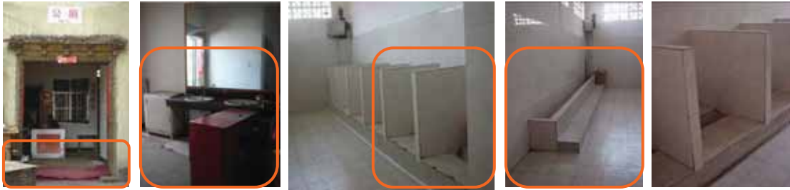
Figure 177: No. 3: Chinese toilet with hold and lower portion in between men and female. There is no toilet for disabled.
