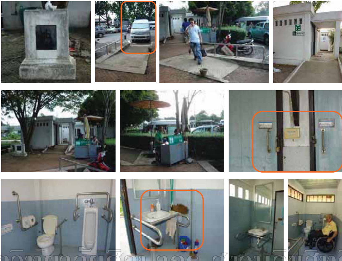
Figure 225: Public toilets for disabled with ramp access open for all users. Major feature is its adaptability to the handicap toilet. However, some other feature does not meet standard such as the entry doors, handle, lock, and storage. The doors do not open for 24-hour access; people have to ask for the key from the superintendent.
