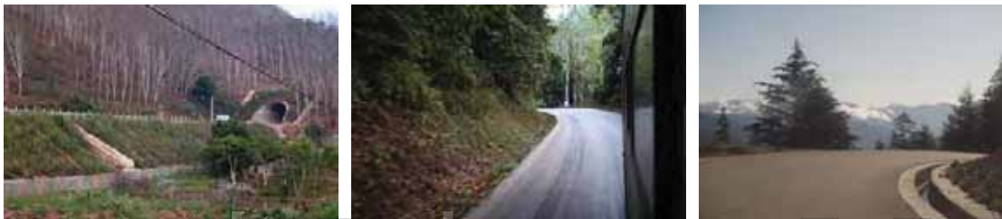
Figure 148: Construction continues on the highway through Lao PDR border to Kunming Yunnan China PRC.
