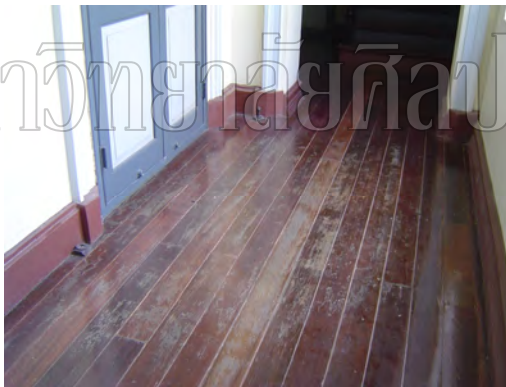
Fig.100 The scratch and peeling of wooden floor Photo by: Supachokeaueychai, T.
