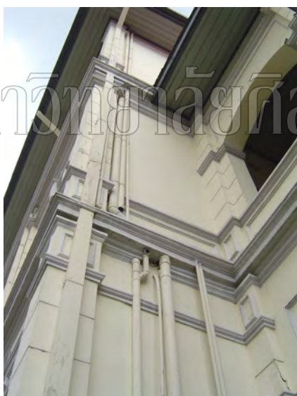
Fig.90 Leakage downspouts cause roofing deterioration Photo by: Supachokeaueychai, T.
