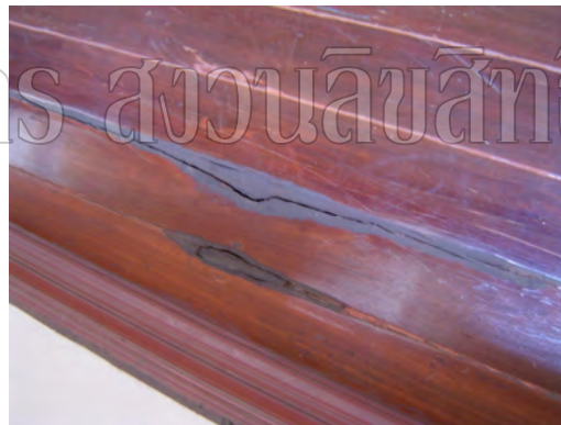
Fig.101 Underground humidity impacted to hardwood flooring
