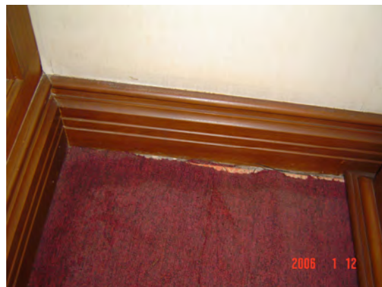
Fig.110 Damp carpet by underground humidity Photo by: Supachokeaueychai, T.
