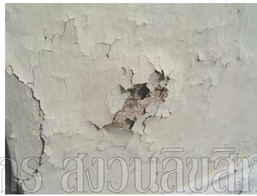
Fig.93 Degradation of masonry wall from water penetration Photo by: Supachokeaueychai, T.
