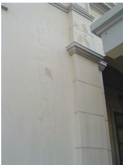
Fig.94 Peeling by incompatible layers of paint emulsion Photo by: Supachokeaueychai, T.
