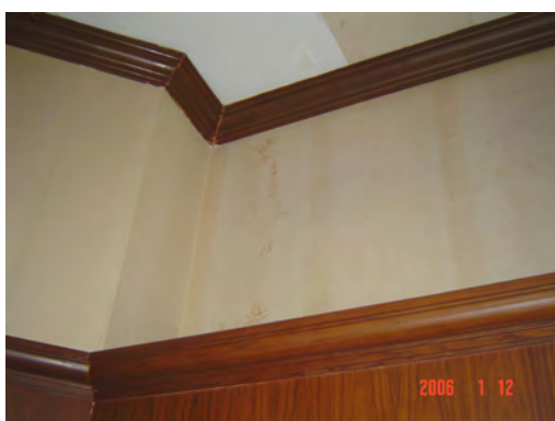
Fig.107 Peeling of wallpaper from Moisture penetration Photo by: Supachokeaueychai, T.
