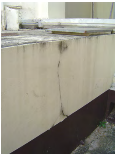
Fig.96 Hair-line cracking of exterior walls Photo by: Supachokeauychai, T.
