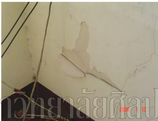
Fig.92 Peeling of paints at the wall Photo by: Supachokeaueychai, T.
