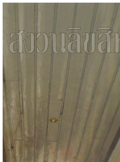
Fig.91 Deterioration by moisture at the exterior ceilings Photo by: Supachokeaueychai, T.
