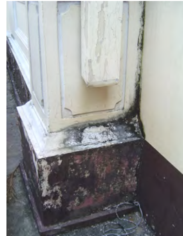
Fig.99 Rising damp from downspout Photo by: Supachokeauechai, T.
