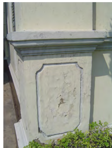
Fig.97 Paint blistering by moisture penetration Photo by: Supachokeauychai, T.
