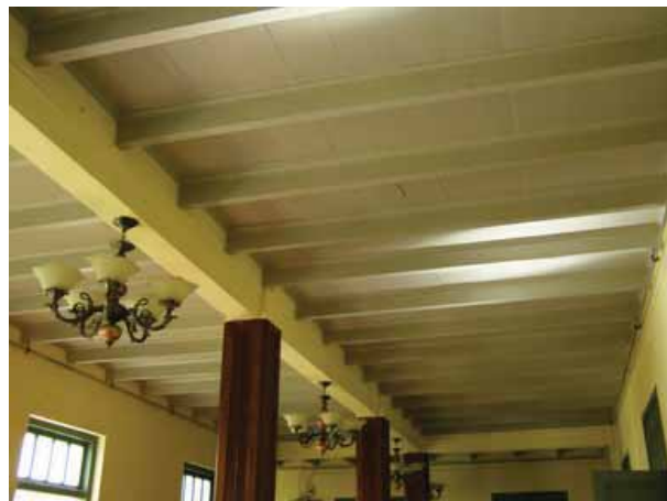
Figure 115: The ceiling that the underside of the floor is exposed showing the supporting wooden joists and the floor planks.
