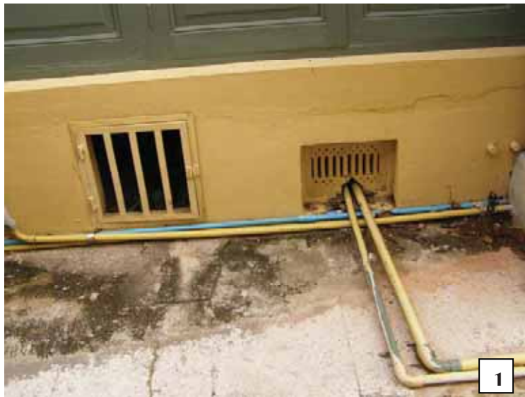
Figure 101: General condition 1 First floor of the building was lifted up 0.80 meters above the ground level and underneath the first floor, there are openings which functions as air vents at intervals around the base of the building.
