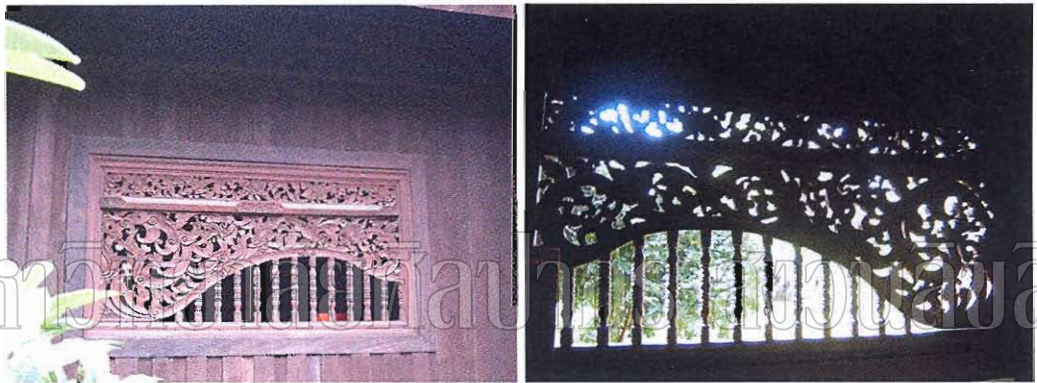
Figure 33 showing the carved wood ventilation grilles from the exterior (left) and the interior (right) of the main building Source: author, 20 August 2006
