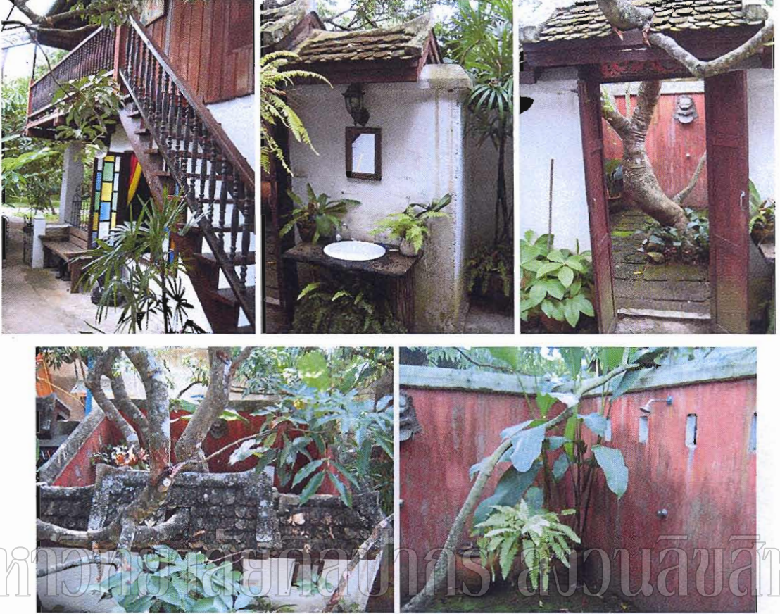
Figure 39 showing the exterior conditions of the secondary building A Source: author, 20 August 2006
