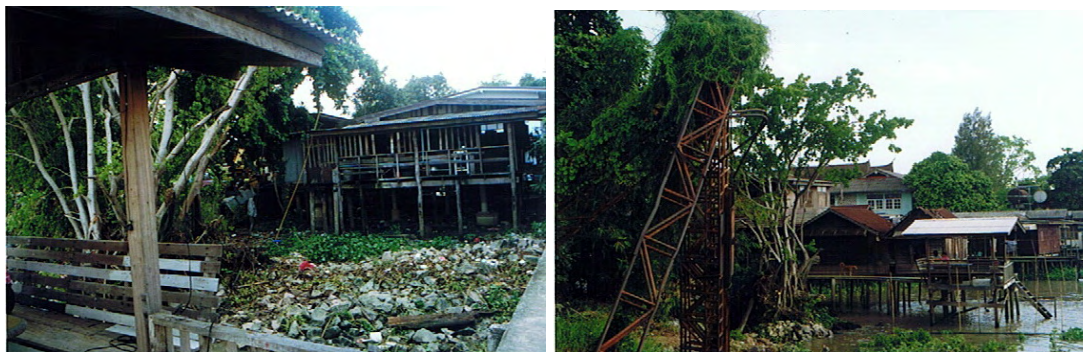
Figure 49 showing the old house of Chamchang Family before adaptive re-use as a restaurant
