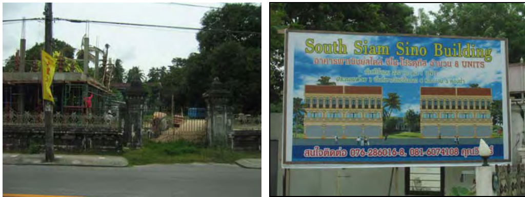
Figure 94 showing the construction and the advertisement of eight units of three-storied shop-houses in front of Ban Chinpracha in September 2008 Source: author, 21 September 2008
