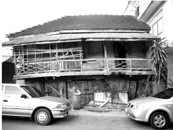
Fig. 27 The poor condition of shophouses along Klong Krasaeng Road. Photograph taken by author on May 2005.
