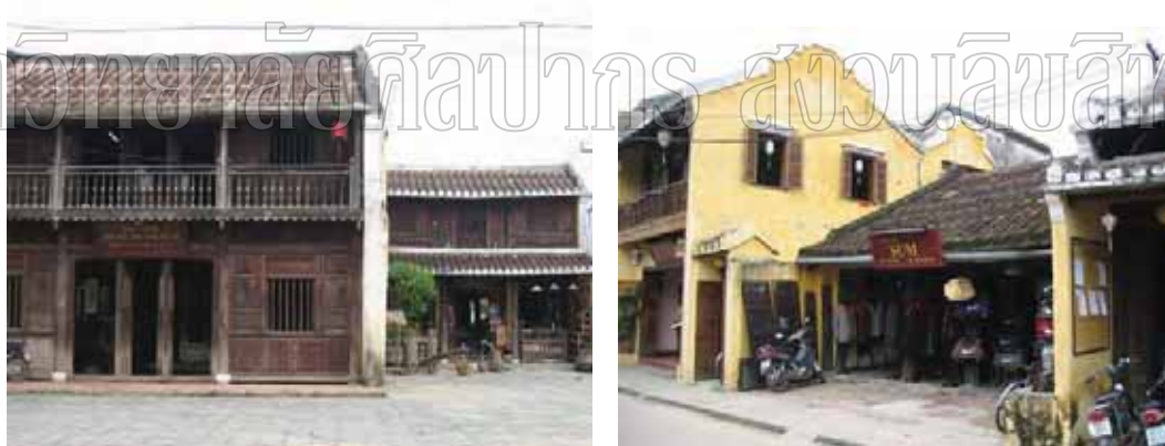
Fig. 49 Since 1993, the emergent roof repair works were carried out on many historical shophouses in the town. Photographs taken by author on 13 December 2006
