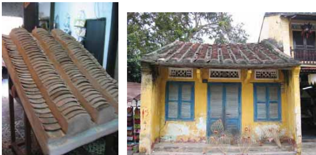
Fig. 48 The restoration process of roof repair works by Hoi An Center for Monuments Management-Preservation. Photographs taken by author on 12 December 2006
