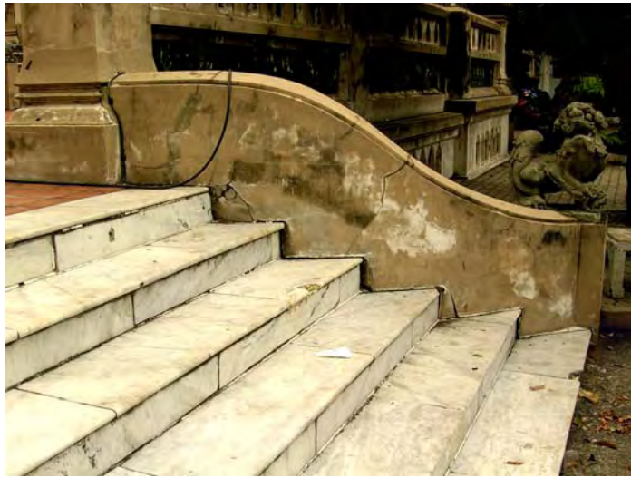
80. The platform of this monastery has small five steps. There are widespread black stains. The plants are glowing between the seams. The tiles are cracked. The floor has sunk.
