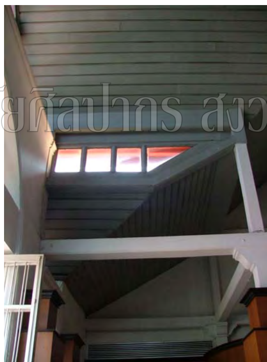
44. The interior view showing the original roof structure of the Phra Thinang Sivamok Pimann
