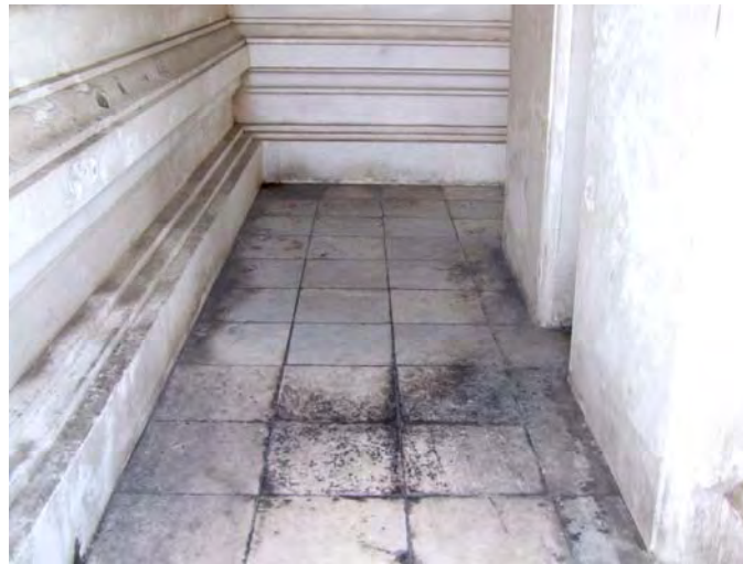
78. The upper basement of this monastery is very dirty because of dirty water.
