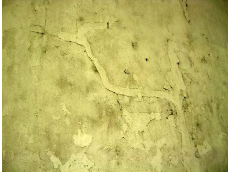
89. Overall the wall is now covered with black stains caused by dampness. Moreover, birds' droppings also affect its original identity and condition.
