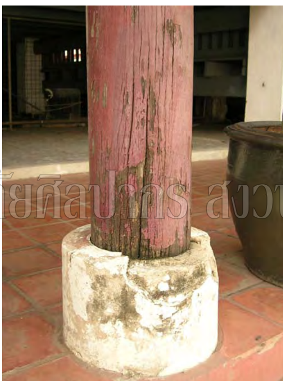
48. The wood pole is split.
