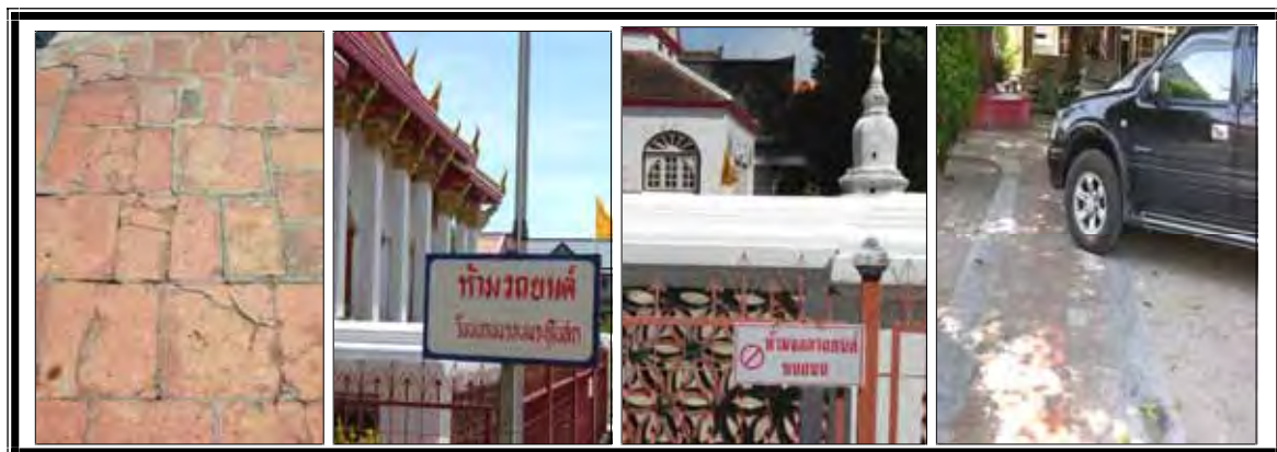
Plate 54 Damaged passageway, the sign posts that prohibit vehicles on the passageway, and parking violation Source: Pensuda Chounchaisit, photograph, 3 April 2007.
