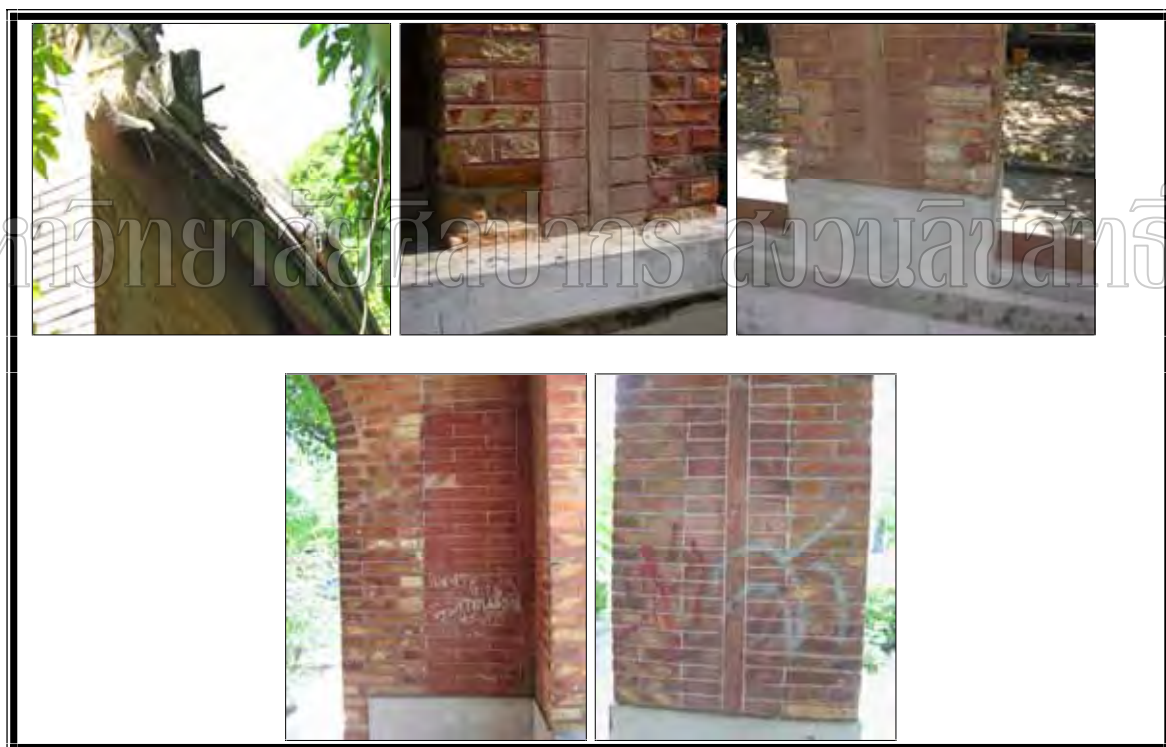
Plate 41 The deteriorations of the hermits' pavilion in the year 2007 Source: Pensuda Chounchaisit, photograph, 3 April 2007.
