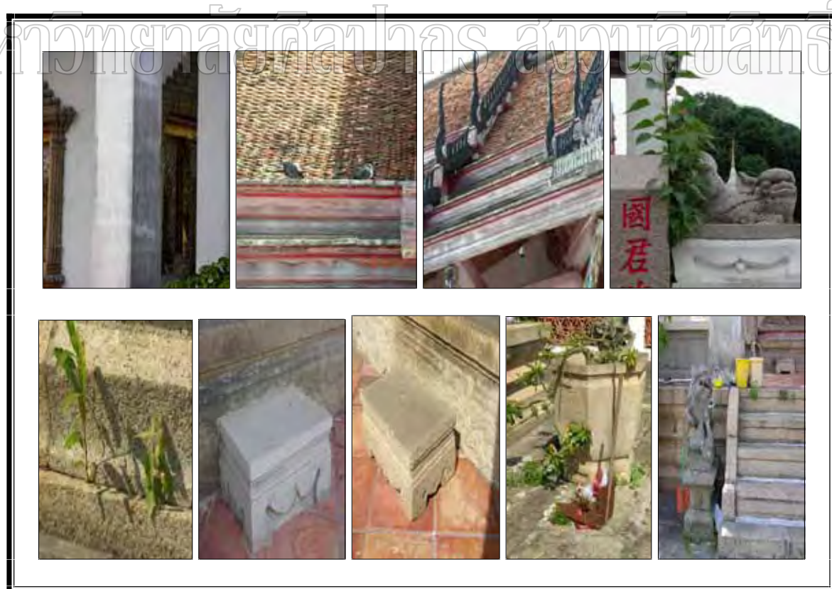
Plate 29 The conditions of the ubosot in the year 2004 Source: Pensuda Chounchaisit, photograph 20 December, 2004.
