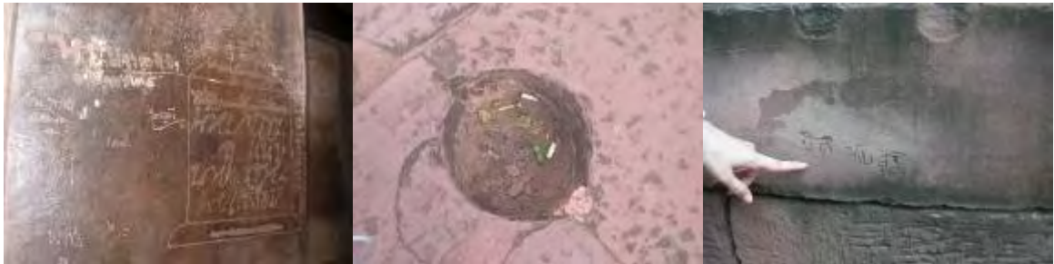
Figure 100: Inside Khmer temples, there were many marks and damages because visitors have not been educated concerning treatment of heritage sites (source: Maneenetr, 2005)
