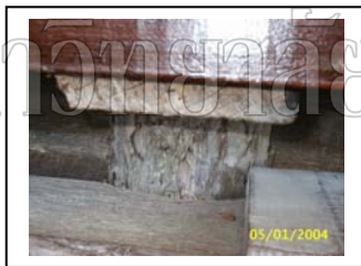
Figure157: Original supporting beam under the ground floor that been attached to raft
