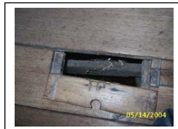
Figure150: A big opening hole at the floor which is used as drainage and repairing hole
