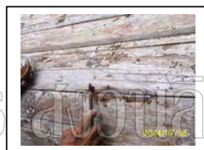
Figure27: Using the mixture of Chan, resin, and red lime fill up at the rotten joint.
