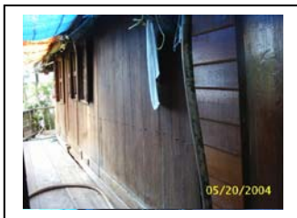
Figure155: External view of wooden wall some parts are new material such as window
