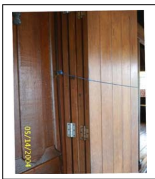
Figure147: Folding door of floating house. In the past, it was a small panel of door.
