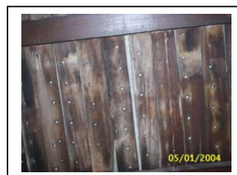
Figure160: Many holes on ceiling were used to fasten thatch in the past.
