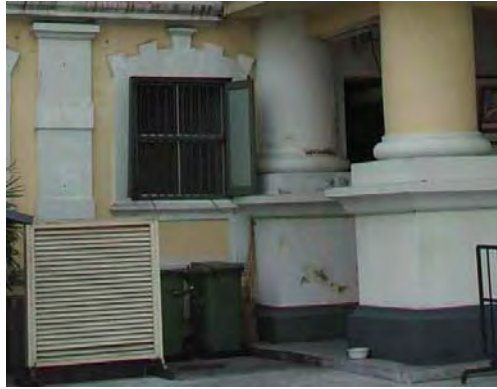
Figure 16. Small cracks and moistures at the base of the column / Building A.
