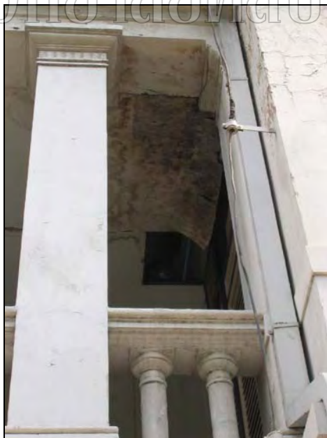
Figure 14 the picture showing the ceiling of the corridor deteriorated by leakage of the roof.
