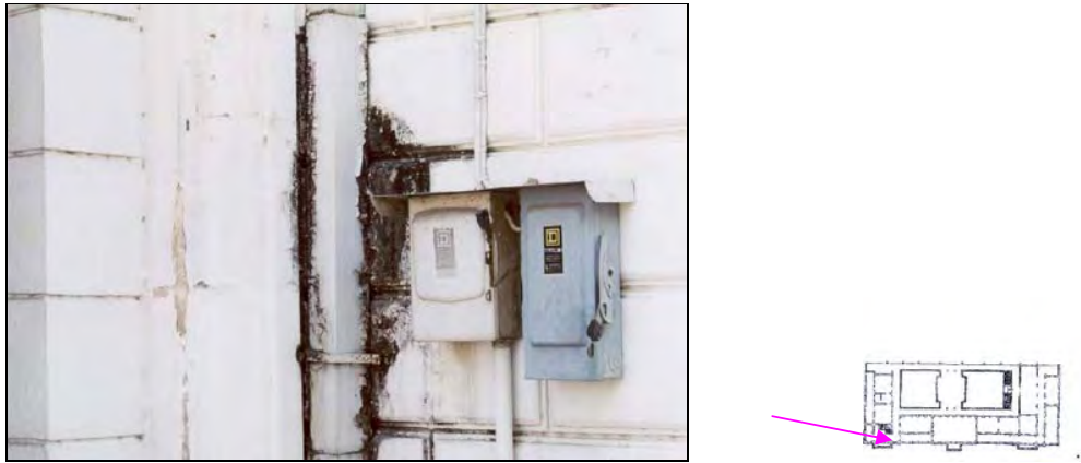
Figure 21 the picture showing the leakage of a downspout next to electrical boxes.
