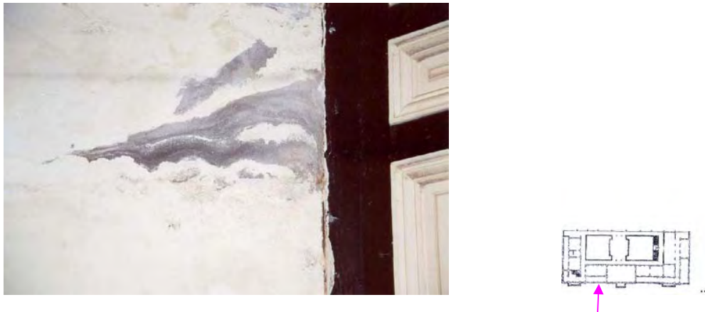
Figure 13 the picture showing the stucco deteriorated by introducing alien materials.
