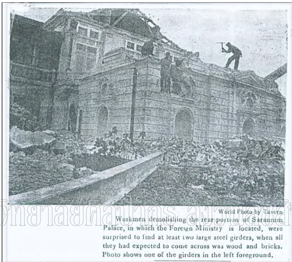
Figure 6 the picture and the article showing the demolition of the front porch of the palace.
