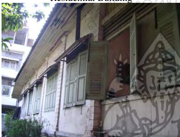
Figure 64 Evidence of moisture and rot on the exterior structure
