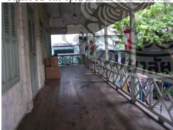
Figure 541 The balcony & the fire extinction hanging on column
