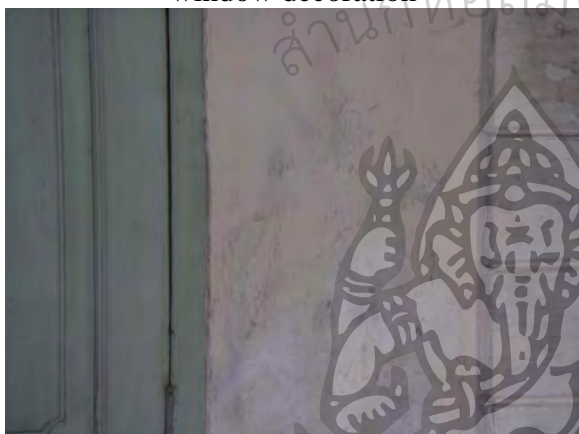
Figure 58 Evidence of moisture and discoloration on the wall (left side on the balcony)
