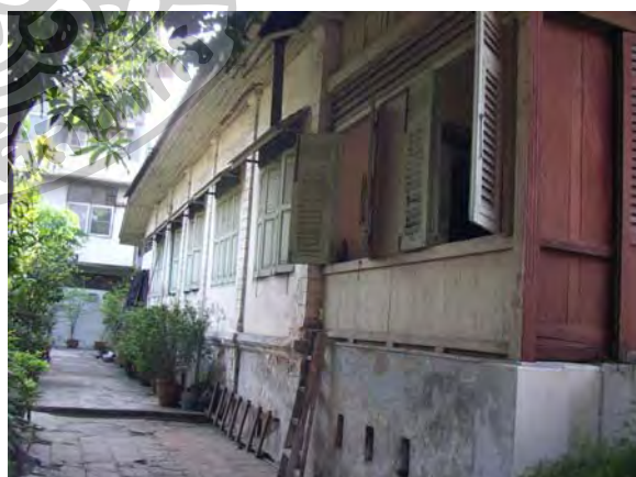
Figure 61 Exterior deterioration on the north side of the Residential Building
