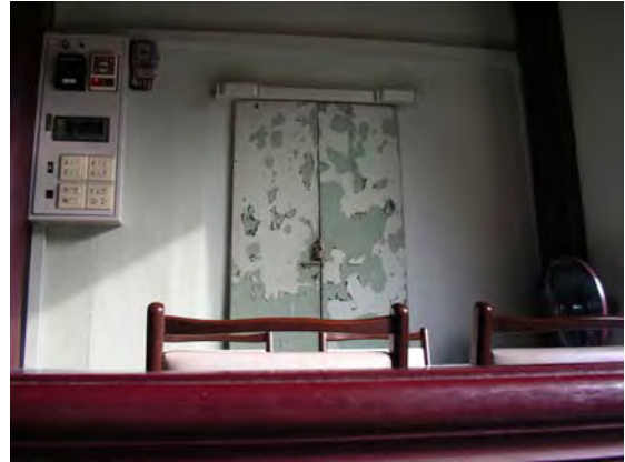
Figure 27 Peeling color on the door
