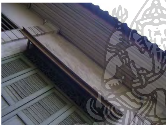
Figure 70 Evidence of moisture on the ceiling
