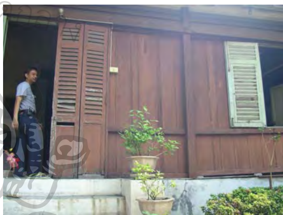
Figure 41 Deteriorate condition of the Residential Building
