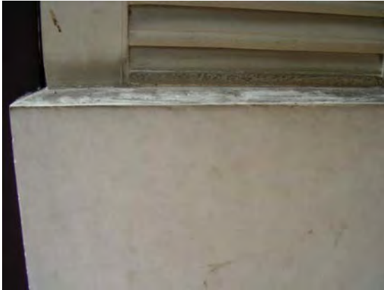
Figure 32 Evidence of moisture
