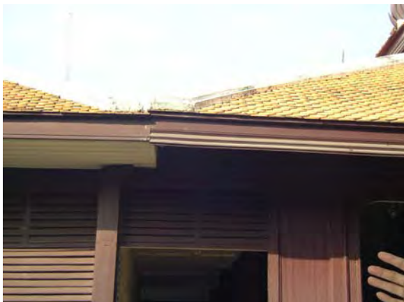
Figure 14 The roof of the original part (on the right) & Additional part (on the left) of the Audience Hall
