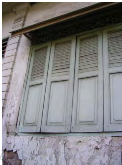
Figure 69 Deterioration of the plaster on the exterior wall
