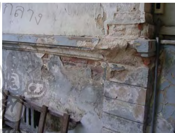
Figure 65 Deterioration of the plaster on the exterior wall
