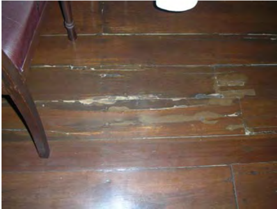
Figure 26 Scratch on the floor
