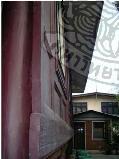
Figure 36 Slightly bent in wall of the Audience Hall
