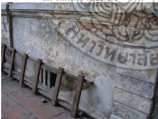
Figure 66 Deterioration of the plaster on the exterior wall
