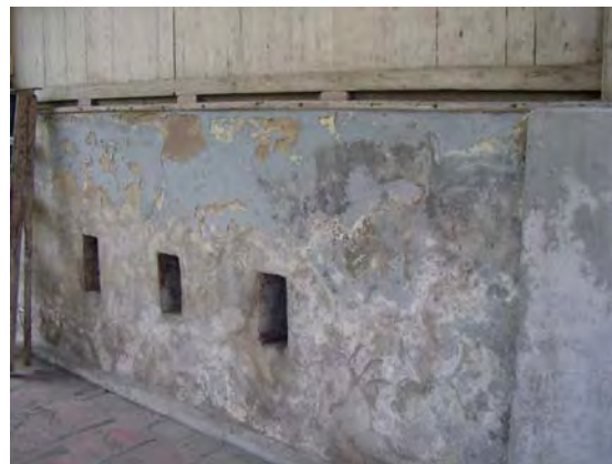
Figure 63 Evidence of moisture at base
