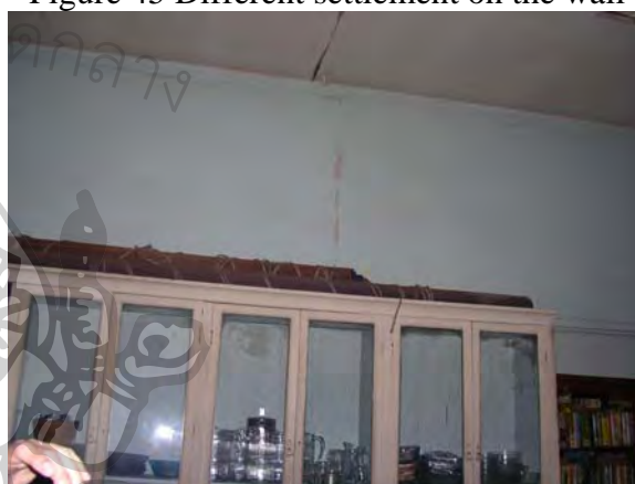
Figure 47 Evidence of moisture from the falling damp on the second room
