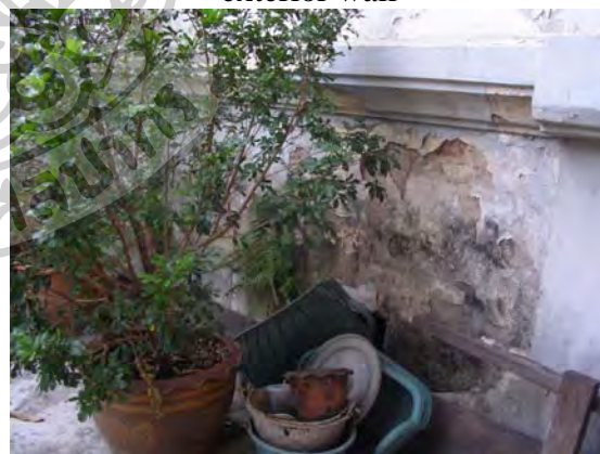
Figure 67 Deterioration of the plaster and fungi on the exterior wall
