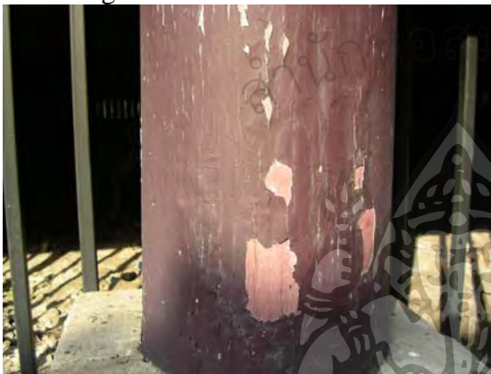
Figure 28 Peeling color & discoloration on the column
