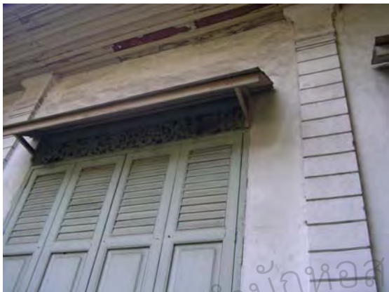
Figure 68 Intact window and rot ceiling
