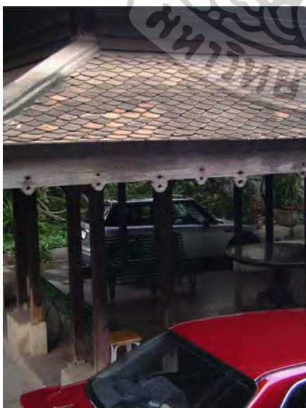
Figure 18 Discoloration on the column of the Wooden Pavilion
