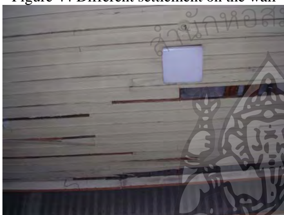
Figure 46 Rot and fungi on the ceiling. Ceiling lighting lamp on the first room ceiling
