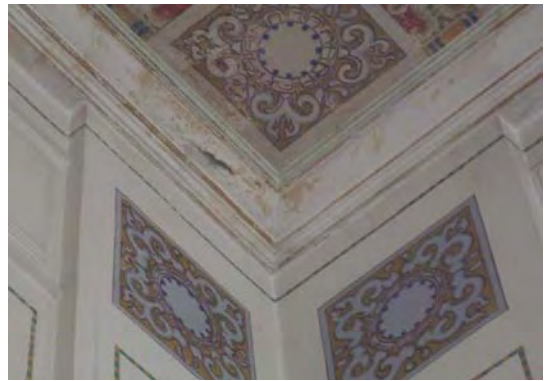
Figure 111 Cracked at the corner of ceiling
