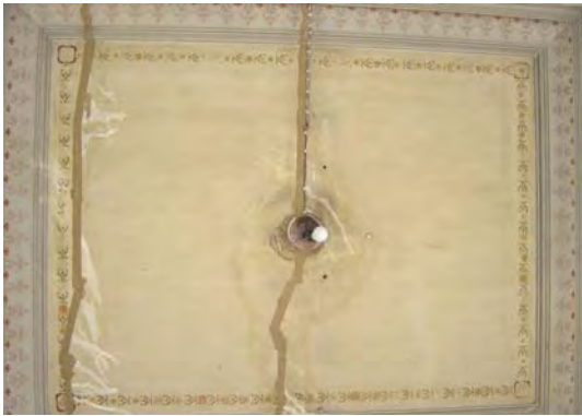
Figure 110 Water leaked from the roof to ceiling.
