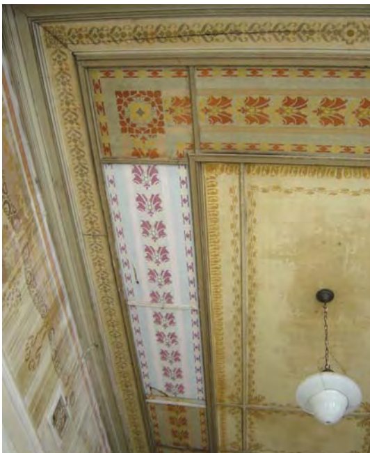
Figure 114 Water leaked from the roof or gutter to the corner of ceiling and wall
