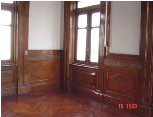
Figure 112 Lacquer was cracked
