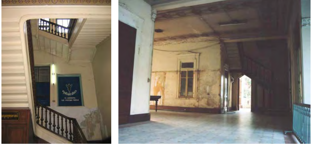
Figure 124 to 125 Colour was cracked and lost
