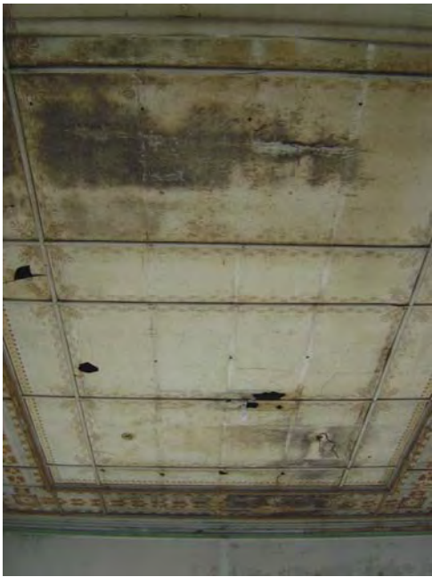
Figure 120 Rot and moldy at the ceiling
