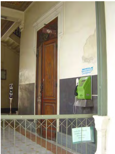
Figure 122 to 123 Colour was cracked and lost
