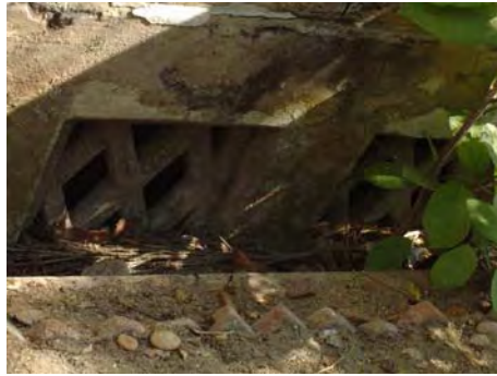
Figure 31 The picture shows the ventilation at the ground floor.
