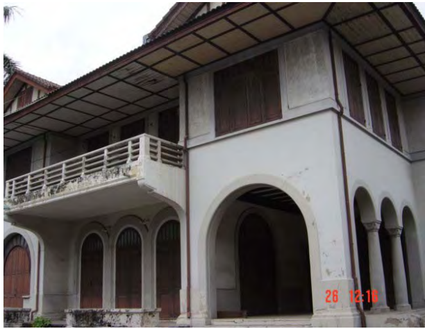
Figure 22 The upper porch with the eave design to suit with the tropical climate.
