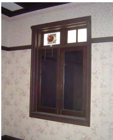
Figure 47 The wallpaper should be taken off since it creates the moist to the building.
