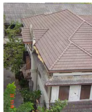
Figure 40 Some area of the roof was destroyed by birds.
