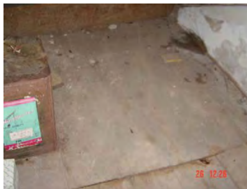
Figure 35: The floor in the storage area was not conserved since the last renovation.
