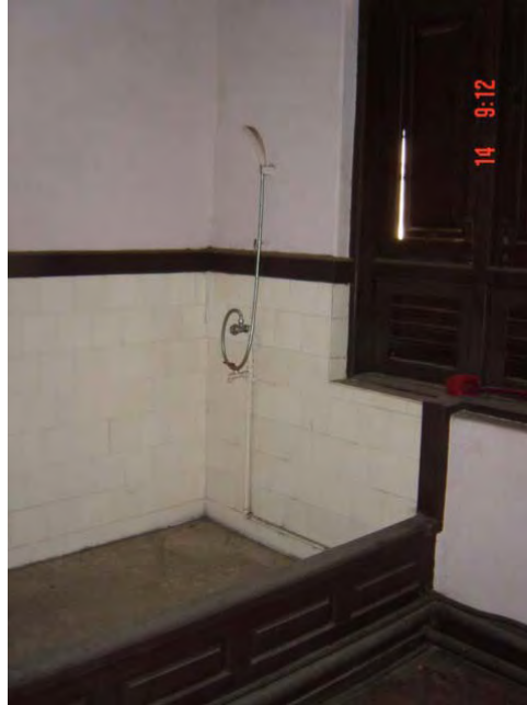
Figure 41 The shower area still remains the original conditions.
