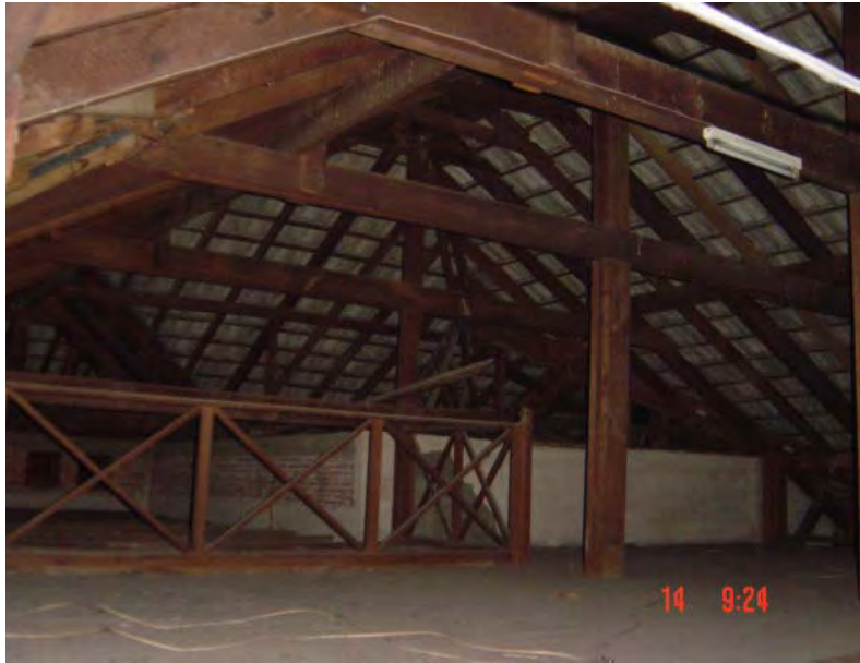
Figure 28 The roof topped was designed to reduce the heat as well as create the space for being the storage.
