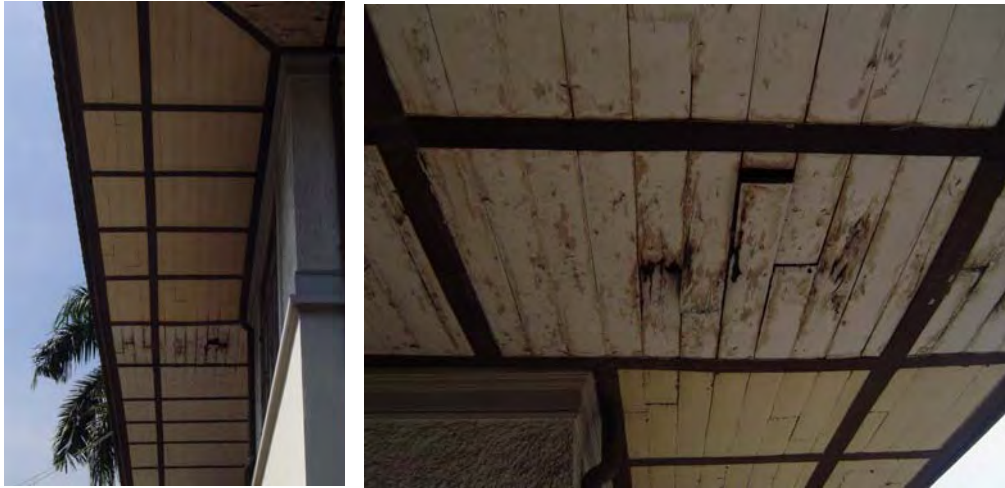
Figure 37 and 38: The ceiling outside the building is rotten in many areas.
