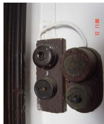
Figure 58 The switches are still remained in original style.
