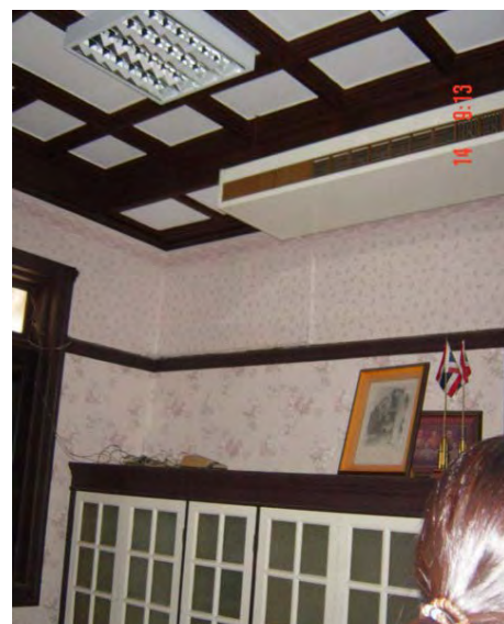
Figure 48 The built-in air conditioning should replace the wall / ceiling types.
