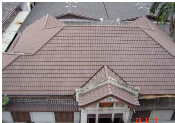
Figure 39 The roof tiles have been renovated without the concern of the issue of originality.
