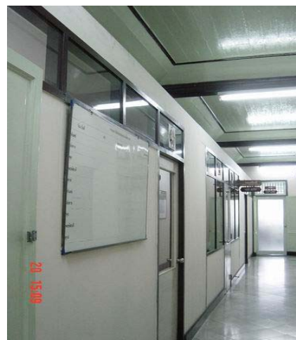
Added room on the terrace. Has gap between ceiling and panel
