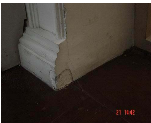
Plaster architrave cracked and scratched, view from the middle room.
