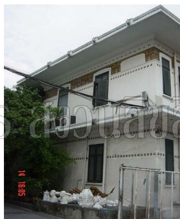
Back of the building near the gate between the Department and Silpakorn University
