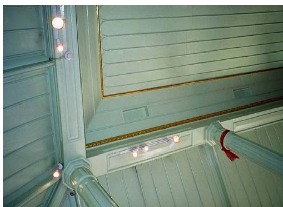
Figure 42 Thong Phra Rong's ceiling, covered with wood, decorated western style, installed track lighting and fire alarm.
