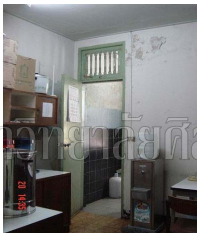
Pantry: the old door remains while new materials were added to wall and floor. Wall has damage of color painted peels and water stains
