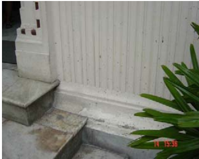
Marble stair in front of the building, has brown stain and dirty surface.
