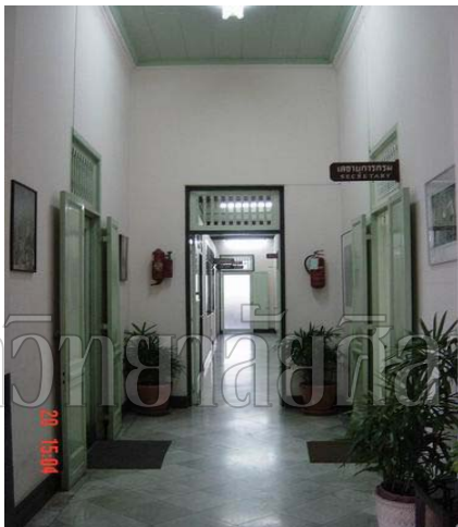
North corridor to the director room in the far end. First room in the east is a gentleman rest room.
