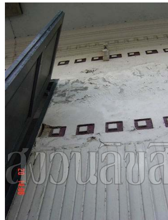
Wall around the upper part of the door. Wall has bad condition such as cracks, exposed cement surface, fungus stains and salt powder.
