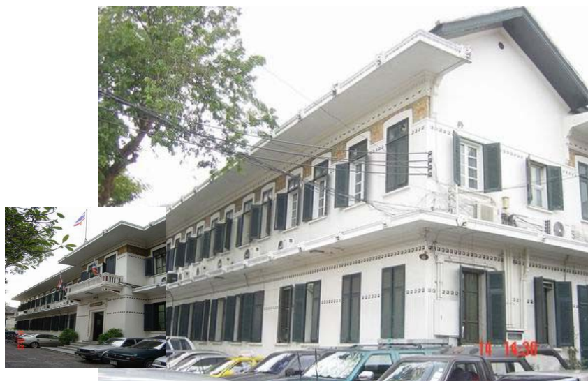
Figure 84 The Department of Fine Arts's building, view from the north. Significant design of the building remains. However, elegance of the building is decreased because of messing electrical wires and air condition equipment.
