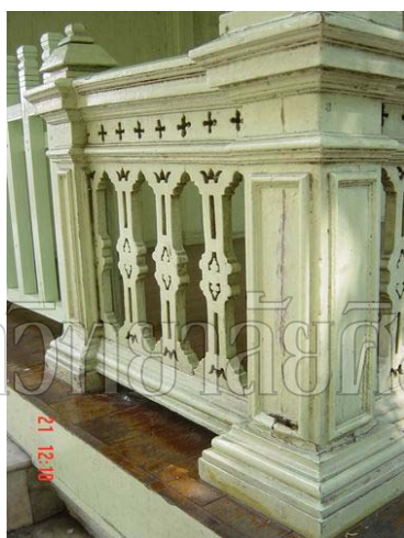
A front column of the pavilion view from the west. This column is in bad condition, wood panel and border are moulded and rotten, it might have insects in side the wood board.
