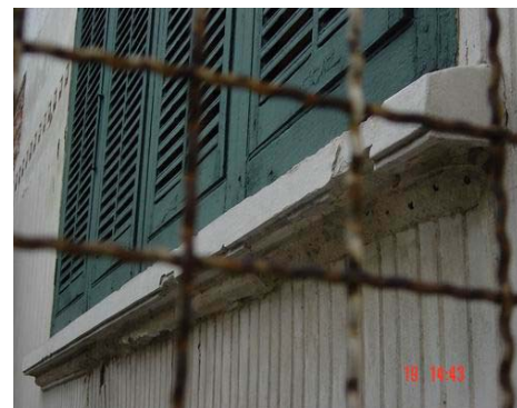
A hornet's nest under the lintel is one of the causes that damage fabric of building
