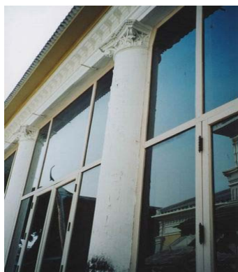
Front of building, decorated with European style plaster moulds. Form and head of column is similar to Tamnak Klang. Between columns added with glass panels and windows.
