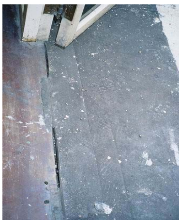
Floor at the door opened to balcony, cracks between rubber sheet and wood floor is a result of raining water leaking into the building.
