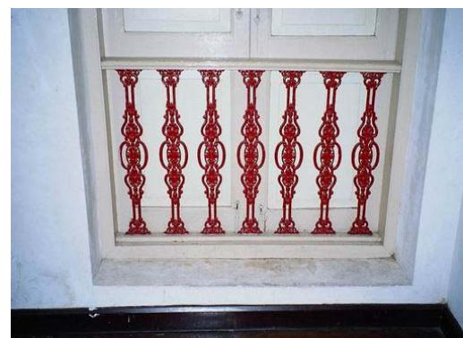
Window at back wall has dry water stain.
