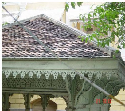
Roof of the pavilion view from the east back. Backed clay roof tiles seem old and decayed, it should be investigated.
