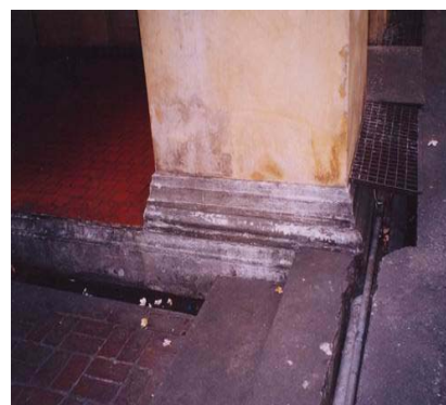
Base of building views from the front. Front and north side of the building has water drains. In the front drain has water in spite of not raining. It indicates drain problem. Base of arch wall and outside cement pavement decay.
