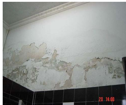
Wall inside lady rest room has damages of painted scratches and peels caused by humid.
