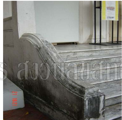
Fungus stains at the edge of the front stair.
