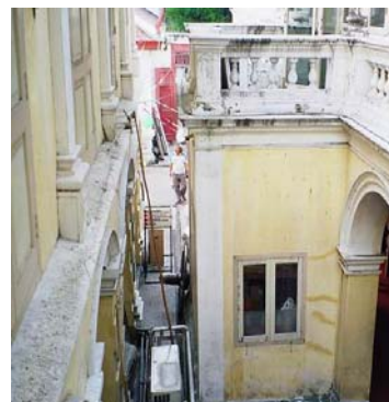
Deterioration of Pannarai building shows clearly. Cracks of walls and stains of fungus and lichen are the major damage of this building. In this picture shows spots of bird's waste on the edge of Tamnak Klang. It is one of many causes of the building deterioration
