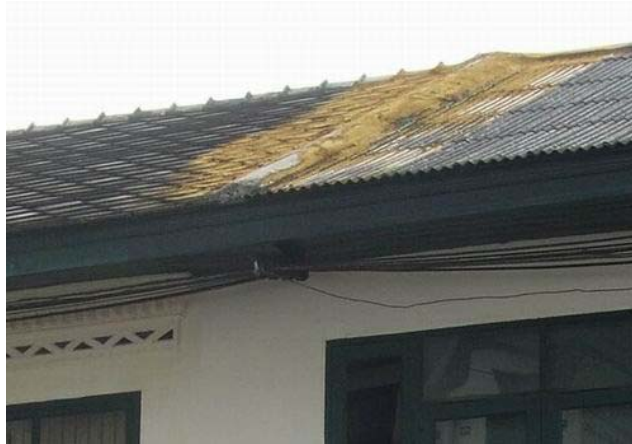
Joint between roof of two parts of building might has some problem of leaking, due to the differential of materials and building constructions
