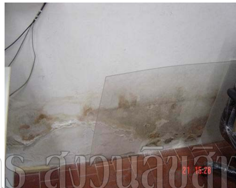
Deterioration of wall in Room no.1, wall stucco cracked and lost. has brown stains of dried water, and powder.
