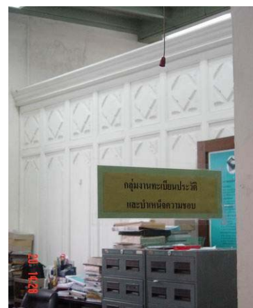
Decorated wood partition in side the room. Cement wall has stains of damp.
