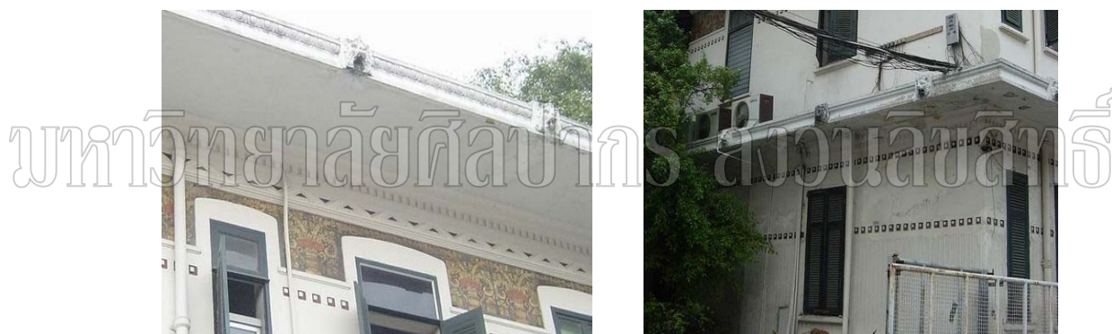
South elevation of the building, upper sunshade has problem of water penetrated, and lion faces rain drains show sign of decays.
