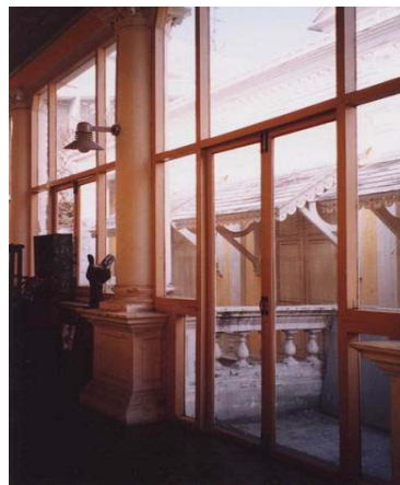
Upper floor balcony has been abandon in bad condition.
