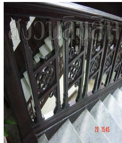
Some detail of wooden rail bar broke and lost
