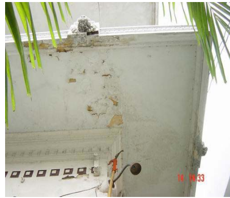
Lower sunshade view north back of the building. Condition of sunshade and wall are bad.
