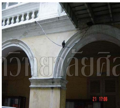
View of the front of Pannarai building under the platform. The plaster arch has been decayed and lost. Disorder main electrical wire has been left carelessly.
