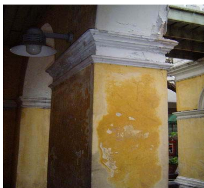
Arch wall of corridor, front of the building, the edge of cement wall and plaster moulding decays. Wall painted discolors and scratches.
