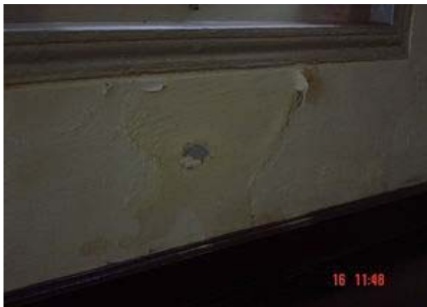
Figure 113 Serious damage of wall inside Thong Phra Rong, view to the wall in the east side. Color painting scratch and peeling in the large stain.
