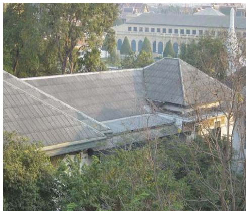
Roof of the Department's office building view from the sixth floor of the faculty of Architecture's building. Joint between roof might have some leaking problem, due to having zinc sheets cover. Added roof over terrace can be identified.
