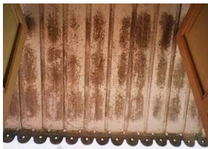
Picture of sunshade, view from inside the building. Below the sunshade, condition of the wood covering is bad, discolor and scattering of fungus stains, for instance.
