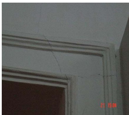
Corner of plaster architrave cracked, view from the middle room.
