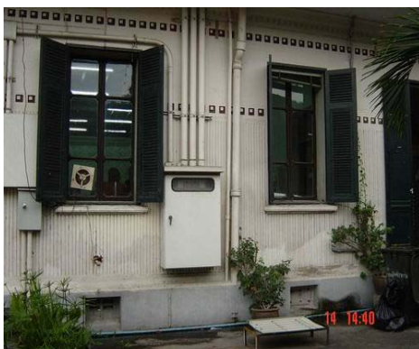
First floor wall in the north side, some electrical equipment was disorder installed. New material was added carelessly, cement block fixed ventilation void at base of building.
