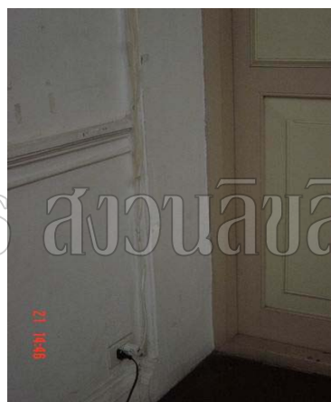
View from inside middle room. The upper floor rooms in this building have poor electrical wire installation and inconvenient uses.
