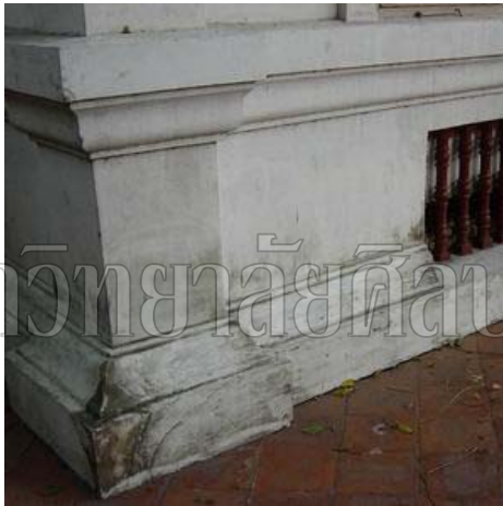
A broken decorated cement at the front elevation.
