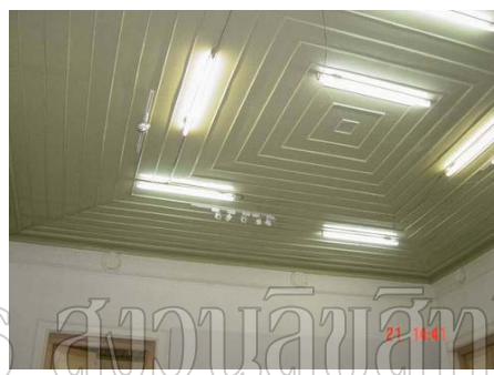
Ceiling of middle room ( Room no. 5 ) has square pattern design different to the other room which are normally straight line of wood board.
