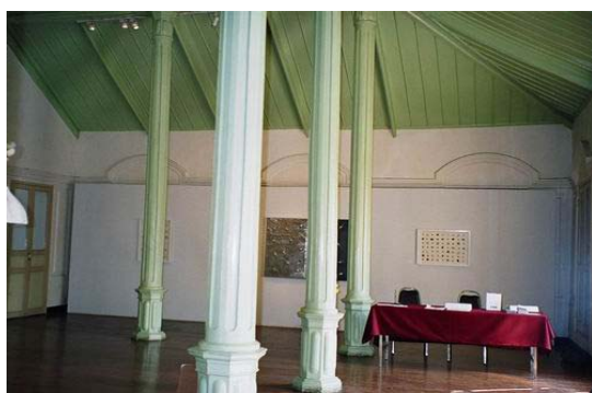
West elevation, decorated wall and windows were covered with gypsum board box for exhibiting paintings.
