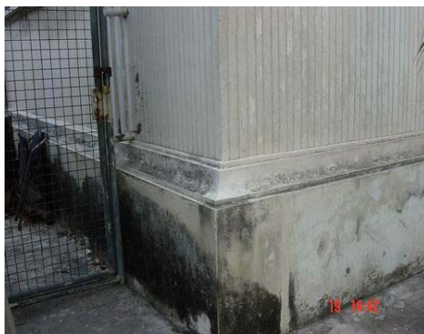
Large fungus stains and color patches, it is occurred by humid from ground water.
