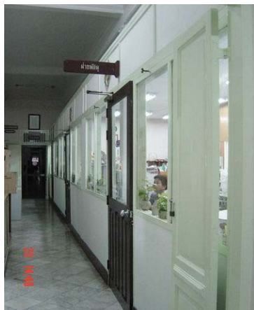
Added office rooms built with light construction. Has gap between ceiling and room partition.
