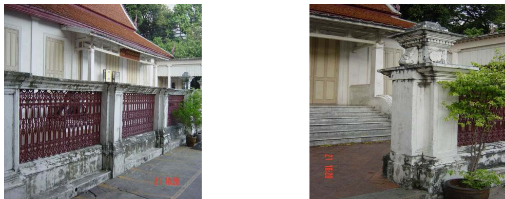
Figure 38 Cement border of Kampung Kaew look old and filthy with fungus stains.
