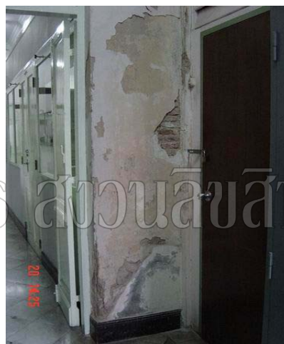
Wall near storage room view from north sub entrance door. Condition of wall is extremely bad. Cement stucco cracked and broke to show bricks construction inside. All the color peeled and has stain of fungus.
