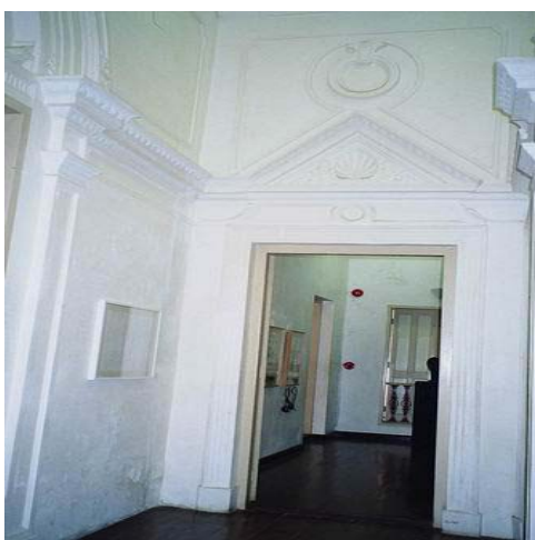
Wall between room no.1 and room no.2, jagged surface and discolor wall can be seen at the lower part of the wall in this picture.
