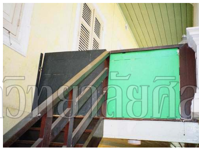
Poor condition of door, View from staircase to upper floor
