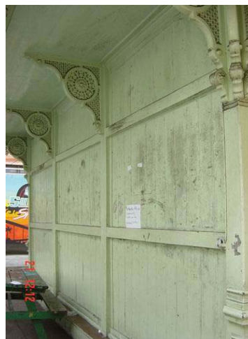
The rare panel view from behind the pavilion. Both sides of board wood panel are full of fungus stains. Color painted scratches and peels. And having inappropriate treat like stick up a notice.
