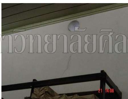
Back wall of storage room behind Room no.4. There are many long hairline cracks on the wall. This problem also happens to the others rooms.
