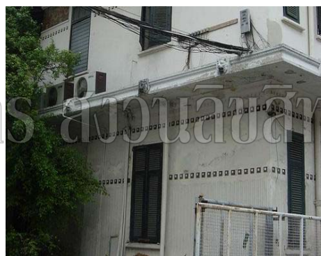
Back of the building, the south side, wall and sunshade are in bad condition.
