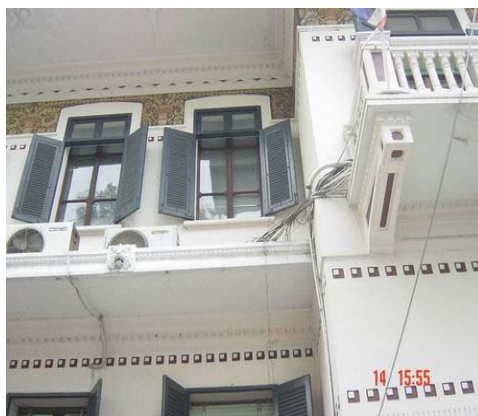
View of front elevation. Careless installation of electrical wires and air condition equipments disgrace the elegance of the building.
