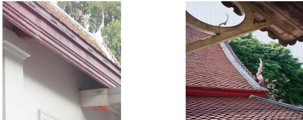
Figure 37 Show condition of roof tile, wooden eaves and cement border. Picture from front side and from back side in the West.
