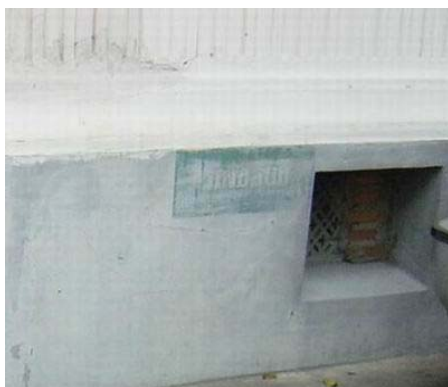
Inappropriate treats to the old building : color screened and ventilation covered. ( efflorescence effect ).
