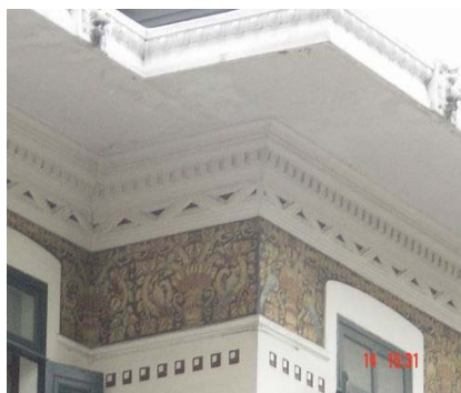
View of decoration details on the upper part of the front elevation. Exquisite fresco painting, graphic plaster moulds, and lion faces at the edge of sunshade are in good condition and clear features.
