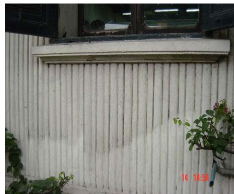
Large water stain on the wall, view from north side of the building
