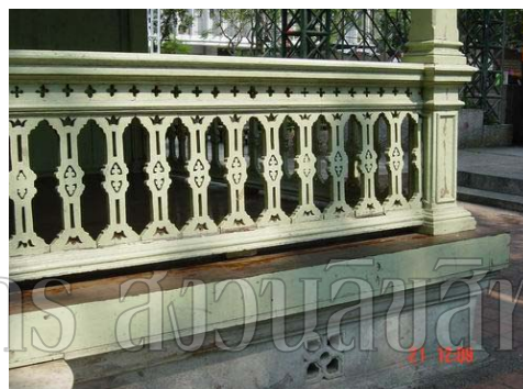
Wood fretwork fence around the pavilion, view from the west side. Condition of wood fence is good. But wood floor and cement base have some damages.
