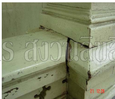
Cracks of wood joints view from the east back column.
