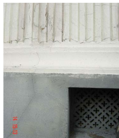
Hair line cracks on the wall, discolor and having powder on the base of building.
