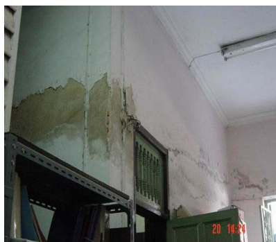
Outside wall of the rest room has bad condition of color peels and stains of fungus.
