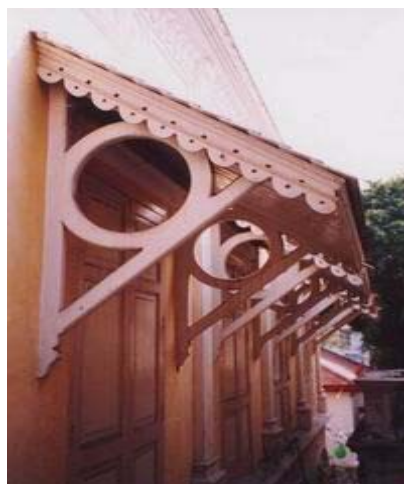
Sunshade over the upper floor window, view from the west. Condition of wood cantilever and eaves are good.
