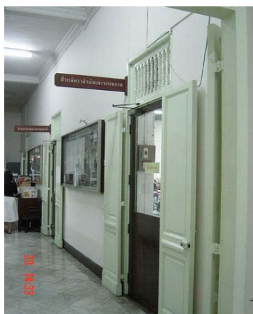
Office room on the front part has old doors with new painted. marble floor like entrance hall.
