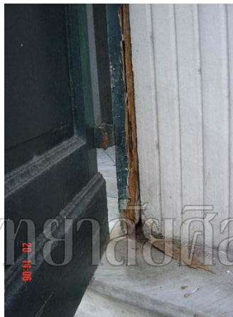
Sub-entrance door on the north side. Door frame cracked and broke in big pieces.
