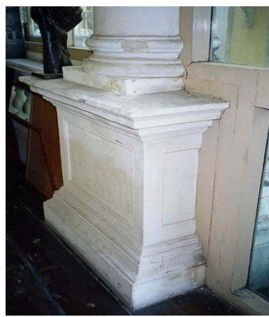
Base of column, view from the door opened to balcony. It has bad condition some part broke and lost.
