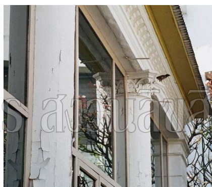
Columns on the upper floor terrace views from balcony. Columns' color painted scratch and peeled.
