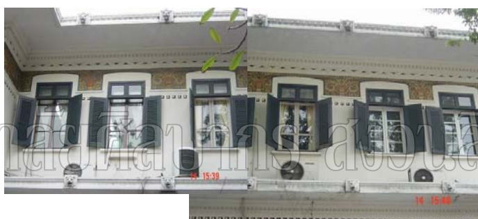
View of front elevation. Varied designs of new added glass windows discourage the beauty of the building.
