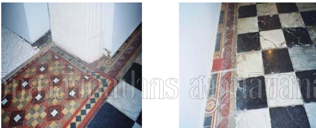
Figure 58 Detail of the old floor pattern in room no.3. In the picture terracotta tile has been replaced where the old tile lost. Those materials seem disunity, it should be replaced by other harmonious material or replica of the original.
