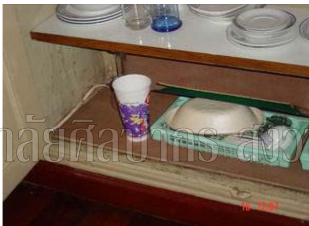
Figure 114 Fungus stain in a pantry cabinet. Cause of problem might be humid or leak of wall or floor of the adjacent toilet.
