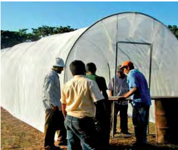
Installation of microtunnel. ST-EP Project: Connecting Local Food Producers and Tourism Enterprises in Nicaragua
